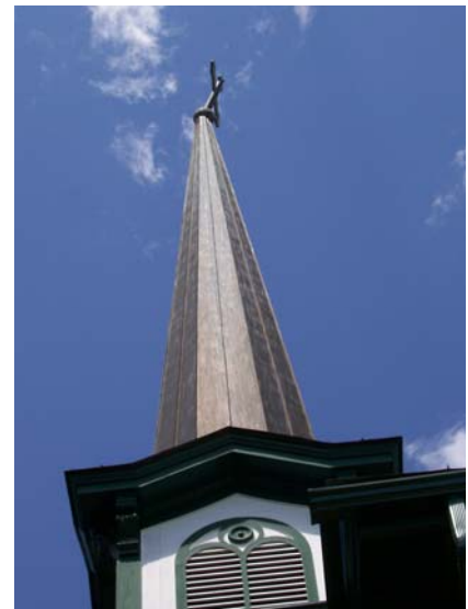
The cross has been repaired, but will never be perfectly straight.
