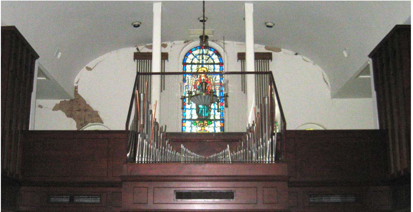
This view is looking up at the balcony, which was now leaning forward. Organ pipes were askew, plaster had broken away from the brick walls, revealing deep cracks and daylight shining through.
